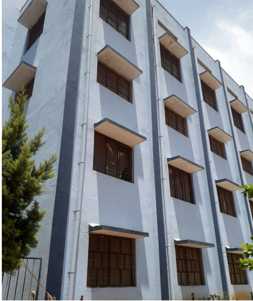
Down pipelines to collect and drain roof top water for ground recharging.
